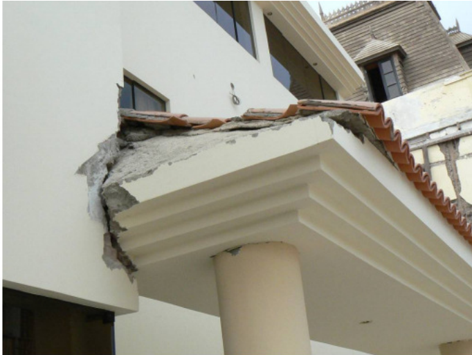
Fig. 3.23. Close up of hotel damage. Relative ground movement, due to liquefaction, between the columns of the exterior roof structure and the building, caused the cracks.
