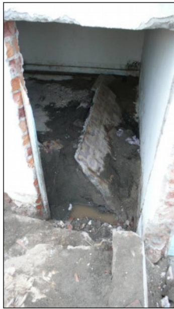
Fig. 3.28. Foundation pushed up due settlement the building.
