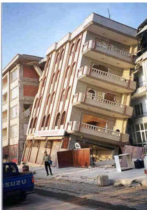
Figure 1: Tilted building due to liquefaction in central Adapazari.
